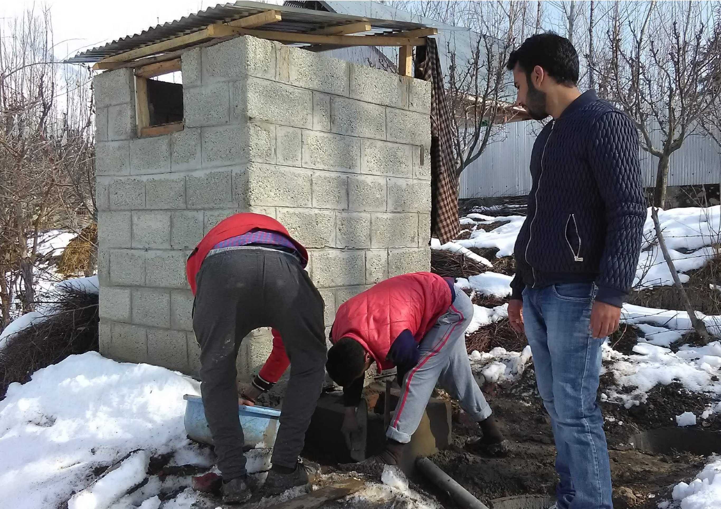
Doctors for You has constructed 538 family toilets in Bandipora Kashmir post floods in 2015
